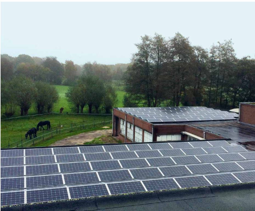
Solar panels - SCHUT PAPIER (Netherlands)
